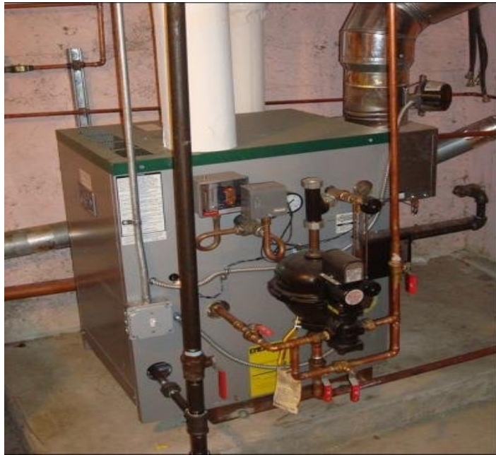
Hot Water Boilers
